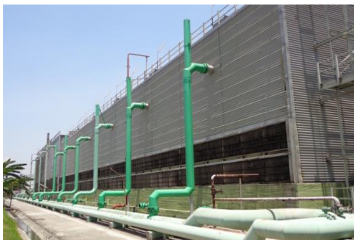
Gambar 1. Cooling tower tipe counter flow di PT Petrokimia Gresik
